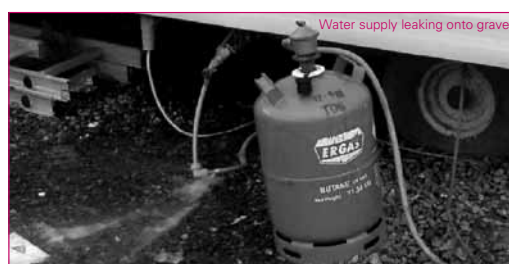
Water supply leaking onto gravel
